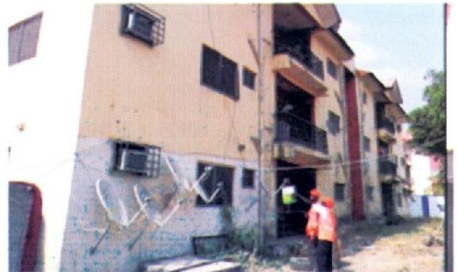
An adjoining similar Block of flats being inspected for possible structural defects by NBRRI and COREN officials
