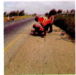
ROAD FAILURE ASSESSMENT
