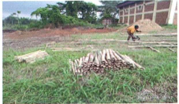
Cutting and Slicing of Bamboo into required sizes for use as pad foundation Mat reinforcements and column starters
