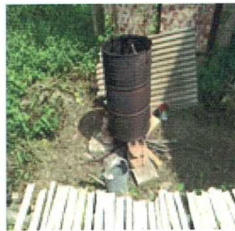
View of a composite starter (steel is used alongside at this level in order to give adequate supporting for the column as Bamboo cannot be bent or curtailed like steel)
