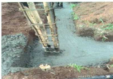
view showing the foundation with starter column being already filled with concrete (mix 1:2:4) and backfilling work in progress
