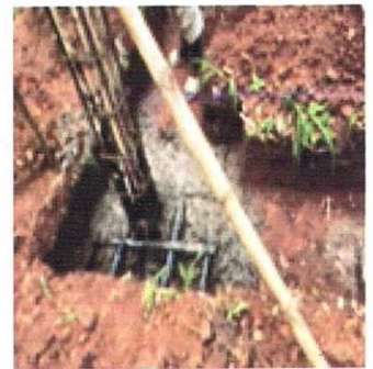
Poured in concrete mix (1:2:4) in the bamboo reinforced column bases in the foundation
