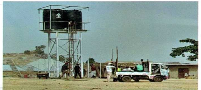
CONSTRUCTED BOREHOLE AT KAFIN KORO COMMUNITY, PAIKORO LOCAL GOVERNMENT AREA, NIGER STATE
