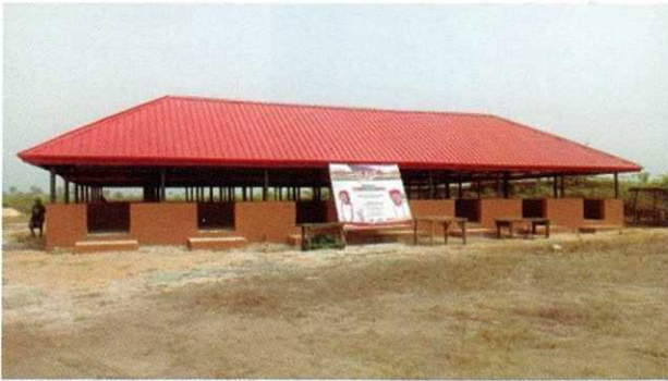
CONSTRUCTION OF NBRRI MODERN MARKET AT AZUNZU, UMUSADEGE, KWALE IN NDOKWA / UKWUANI FEDERAL CONSTITUENCY, DELTA STATE
