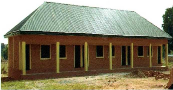
DEMONSTRATIONS OF BLOCK OF THREE (3) CLASSROOMS WITH OFFICE AND FURNITURE AT DIFFERENT LOCATIONS (BENUE STATE)
