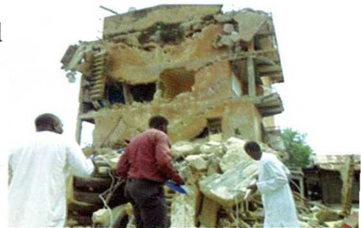
Building Collapse Investigation at Kubwa, Abuja
