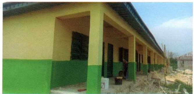
CONSTRUCTION OF TWO NOS BLOCK OF 6 CLASSROOMS EACH WITH SEPARATE TOILETS FOR FEMALE AND MALE STUDENTS TEACHERS AT EFFRUN-OTOR, SECONDARY SCHOOL, UGHELLI SOUTH LGA, DELTA CENTRAL SENATORIAL DISTRICT
