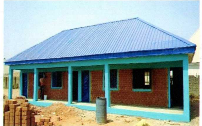
RENOVATION OF PF LUKEMAN ISLAMIYA (LEA) PRIMARY SCHOOL, LAFIA (LEA PRIMARY SCHOOL, REFUGE CAMP, LAFIA)
