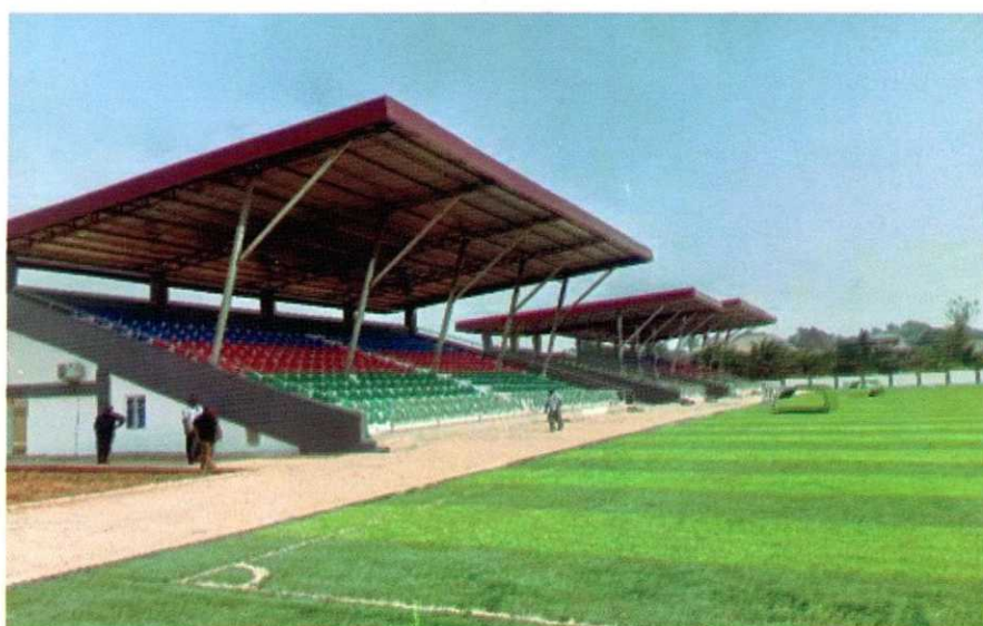
CONSTRUCTION AND REHABILITATION OF TOWNSHIP SCHOOL II STADIUM IN IGBO-EZE SOUTH LGA, ENUGU STATE
