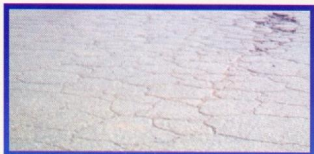
High severity Alligator cracks on the pavement
