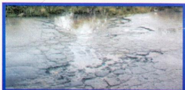
Structural failure due to poor drainage design at the foot slope of the road
