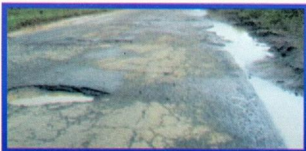
Poor drainage design and lack of routine Maintenance
