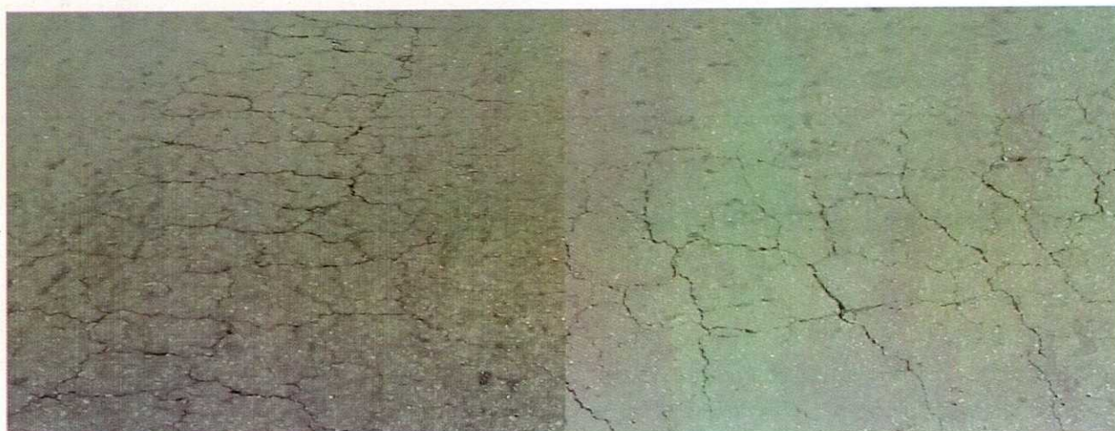
Plate 1: Fatigue cracks observed at various sections along the roadway
