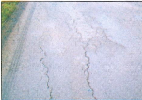
PLATE 11: Moderate severity longitudinal cracks on the wheelpath of the road
