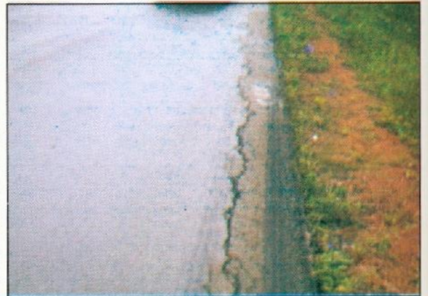
PLATE 12: Low severity longitudinal crack at the edge of the road
