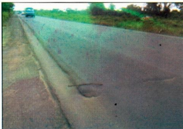
PLATE 6: Typical potholes at the centerline of the pavement
