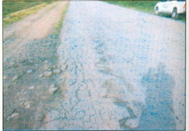
PLATE 10: High severity longitudinal cracks on the edge of the pavement due to undercutting by erosion, Enugu Bound lane
