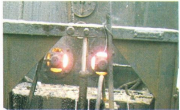
Photo 12 – Heating bitumen and kerosene to the required temperature to produce tack coat or MC1
