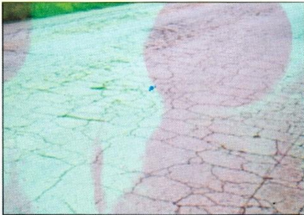
PLATE 4: High severity alligator cracks
