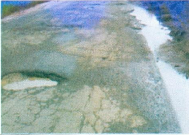
PLATE 7: Poor drainage design and lack of routine maintenance
