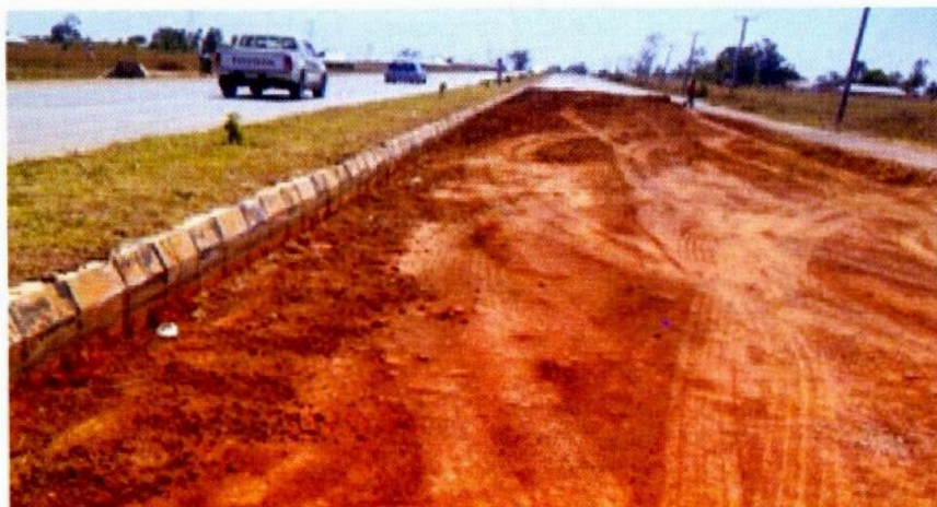
Figure 11: Pavement Failure during Construction
