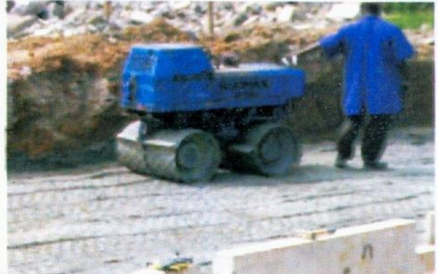
Photo 37 – Compacting stone base using sheep's foot vibratory roller (Courtesy: Julius Berger Nig. Ltd.)
