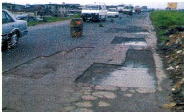
Photo 33 – Selective scarification of pavement sections. Areas not scarified will not be repaired.
