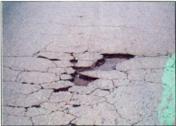
PLATE 3: High severity alligator cracks with the loosening of the pieces of asphalt
