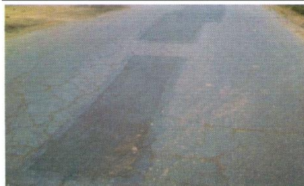
Photo 34 – Bird's eye view of rehabilitated road section. Note the existence of medium severity alligator cracks around rehabilitated area
