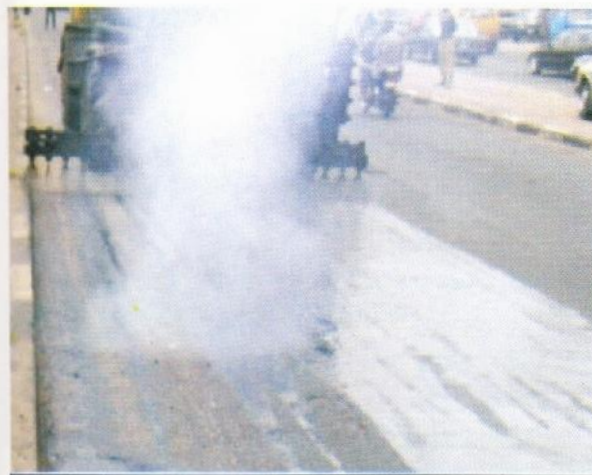
Photo 13 – Bitumen heater spraying tack coat on existing pavement. Notice the many gaps
