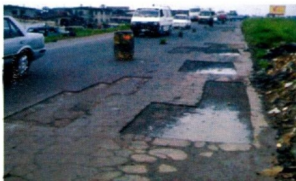
Photo 33 – Selective scarification of pavement sections. Areas not scarified will not be repaired.
