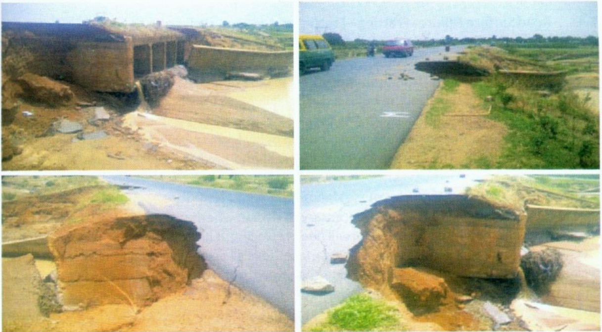
Figure 10: Failed Roadways due to Erosion and Poor Drainage
