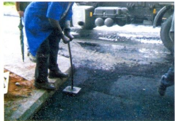
Photo 43 – Using hand rammer to compact tight area not easily accessible to roller (Courtesy: Julius Berger Nig. Ltd.)
