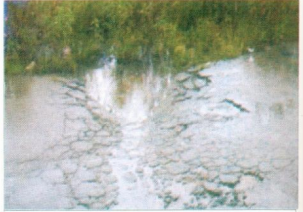
PLATE 8: Structural failure due poor drainage design at the footslope of the road
