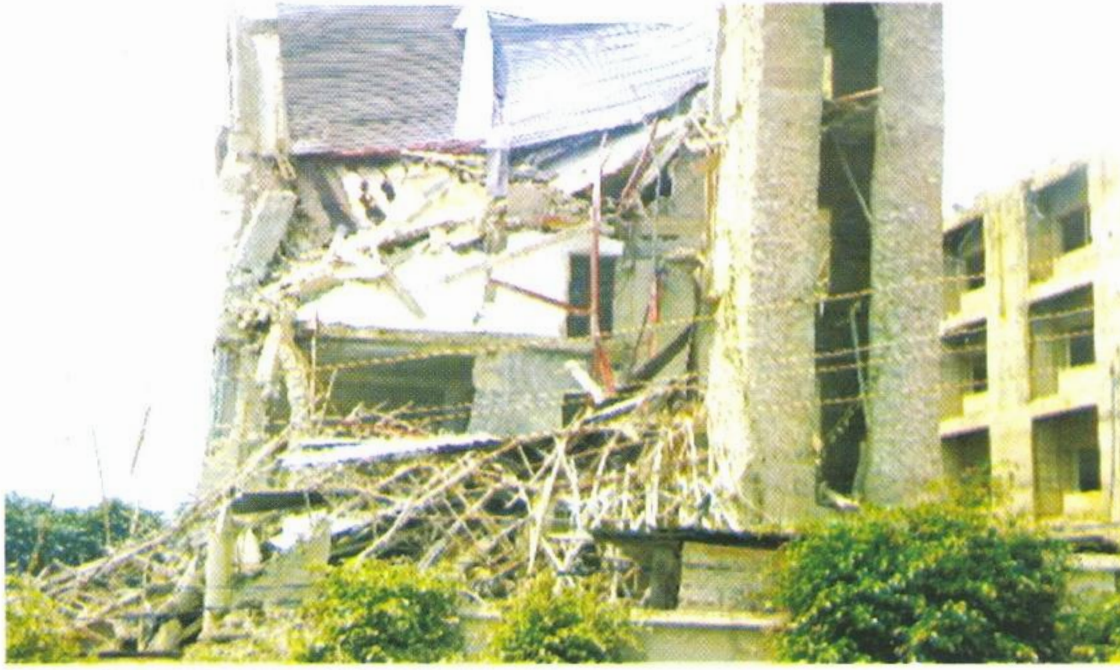
PLATE 9: PARTIAL COLLAPSE OF SIX (6) STOREY BUILDING AT PORT-HARCOURT STREET GARKI 2, ABUJA
