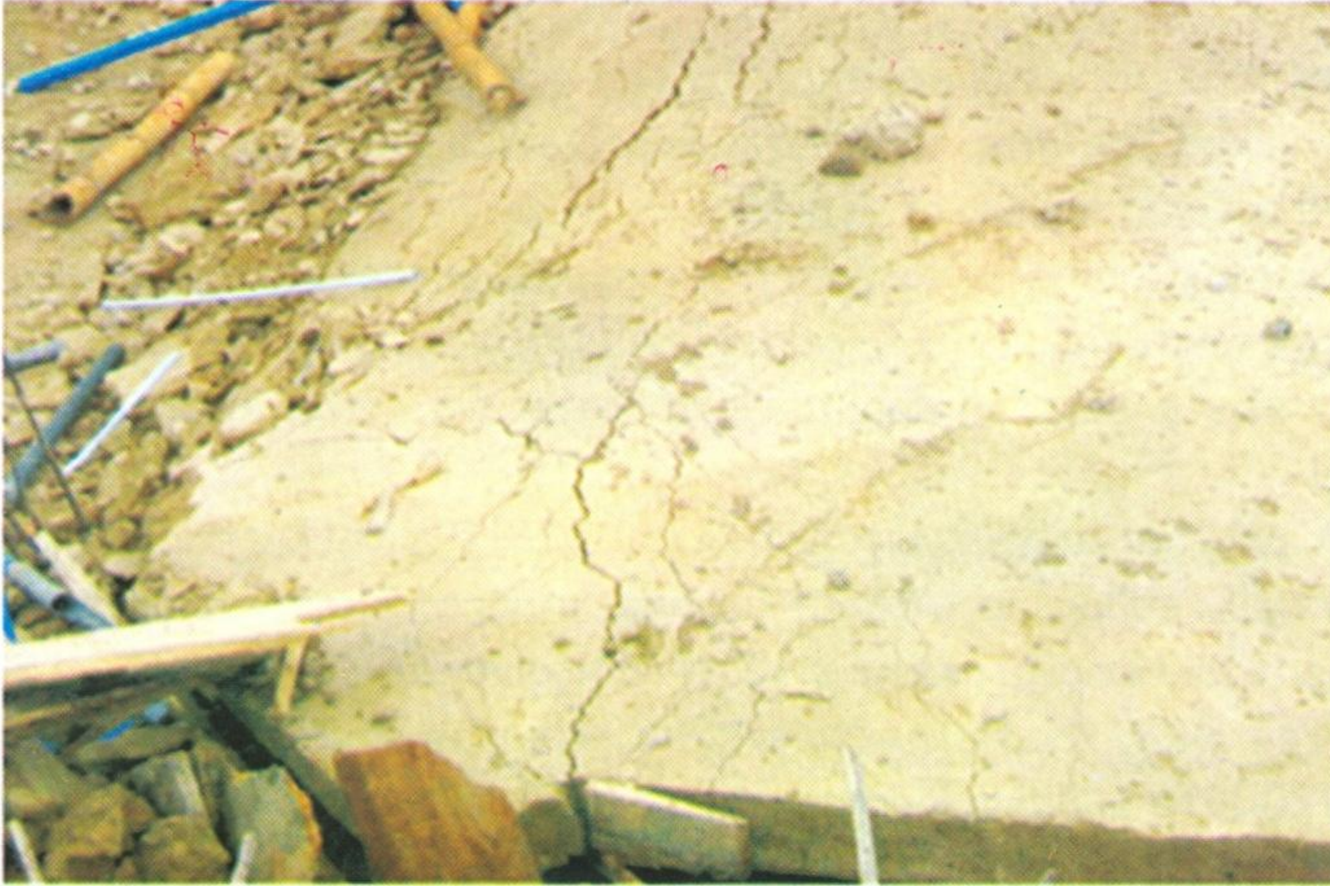
PLATE 1: A COLLAPSED HOTEL BUILDING IN AKURE.
