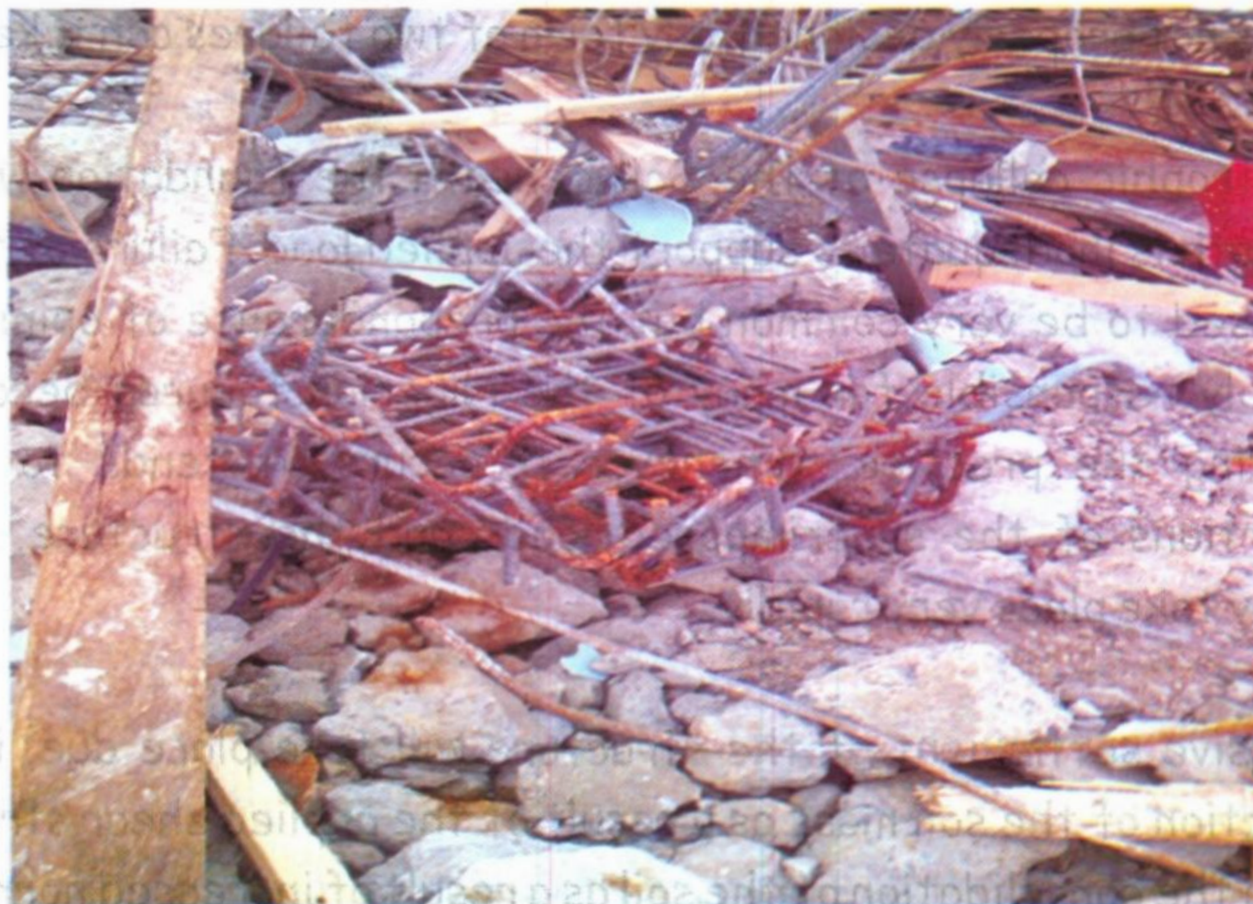
Figure 6: Mararaba Collapsed Site Showing Footing Reinforcement clearly under-sized (450mmx450mm)
