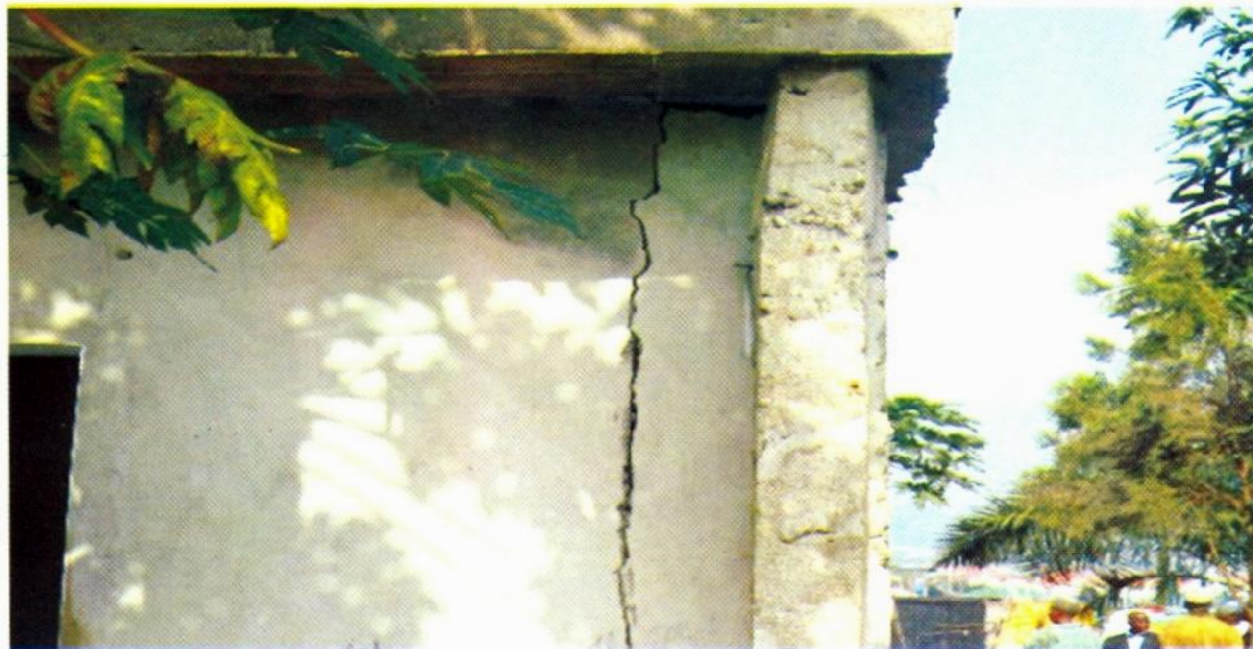
PLATE 12: CRACK ON THE BUILDING DUE TO DIFFERENTIAL SETTLEMENT IN GWARIMPA FHA, ABUJA
