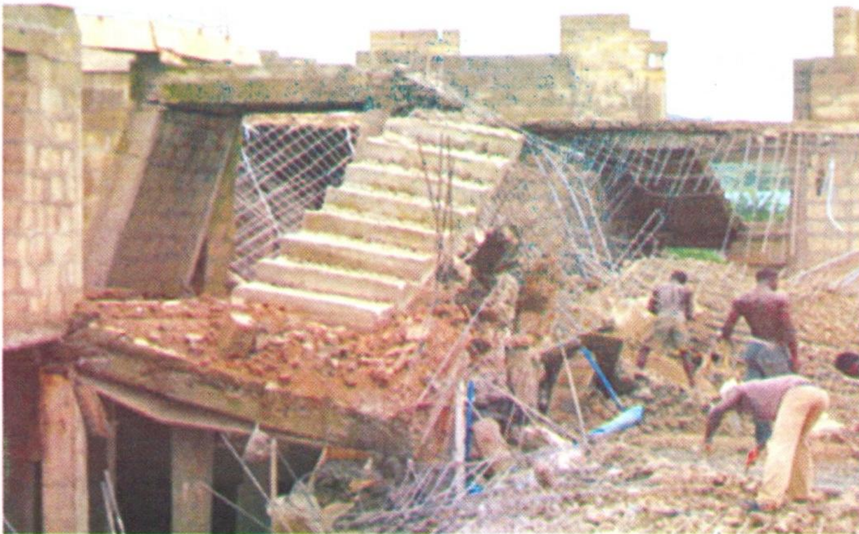
PLATE 2: A COLLAPSED HOTEL BUILDING IN AKURE
