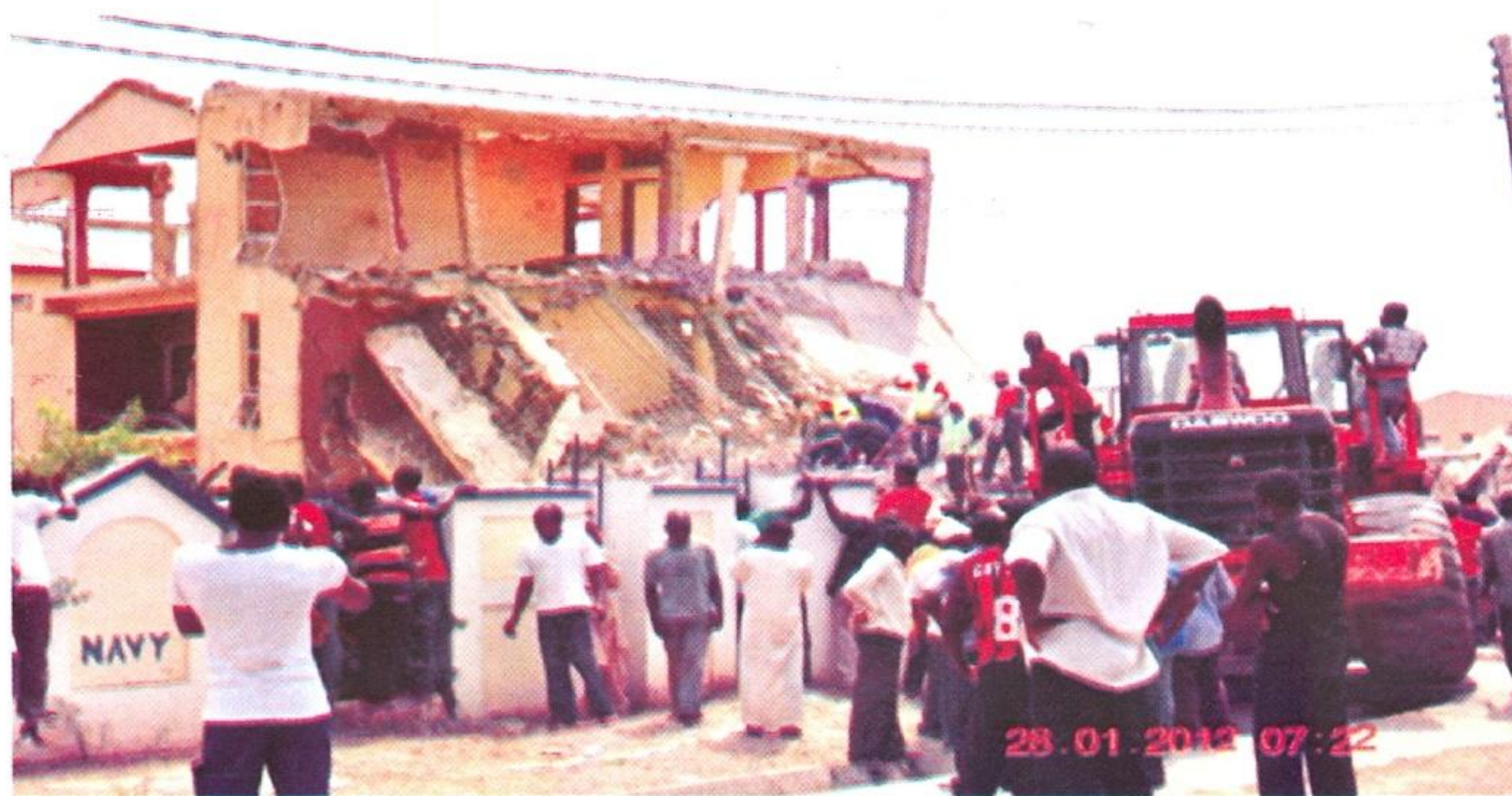
PLATE 8: COLLAPSE OF A TWO STOREY BUILDING OWNED BY NIGERIAN NAVY IN GWARIMPA, ABUJA
