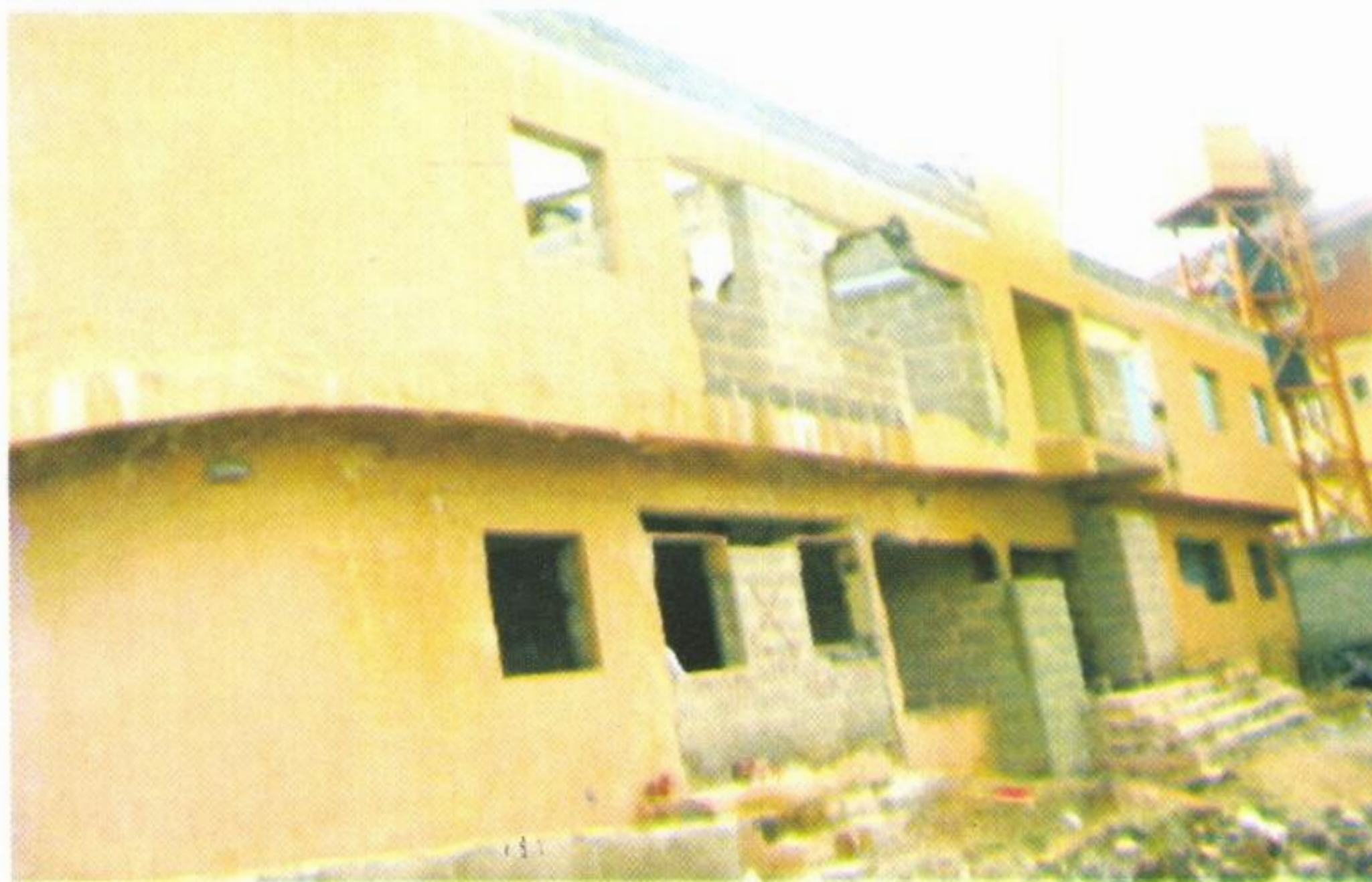
PLATE 10: DEVELOPER INCREASING THE HEIGHT OF BUILDING WITHOUT RECOURSE TO THE AUTHORITY
