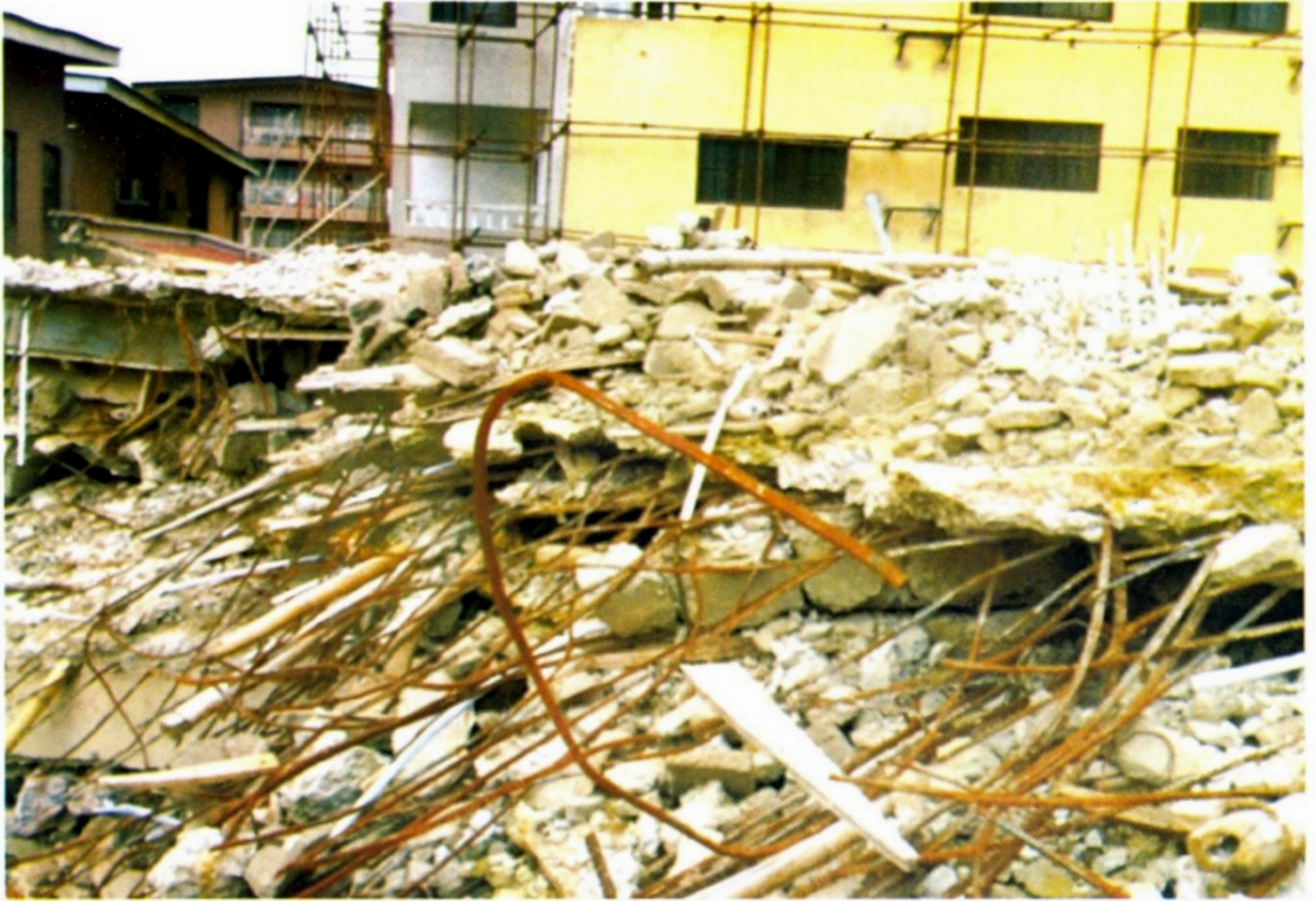
Figure 1: Collapse of 5-storey Hotel under construction at Adenubi Close, Ikeja - Lagos, March 2011
