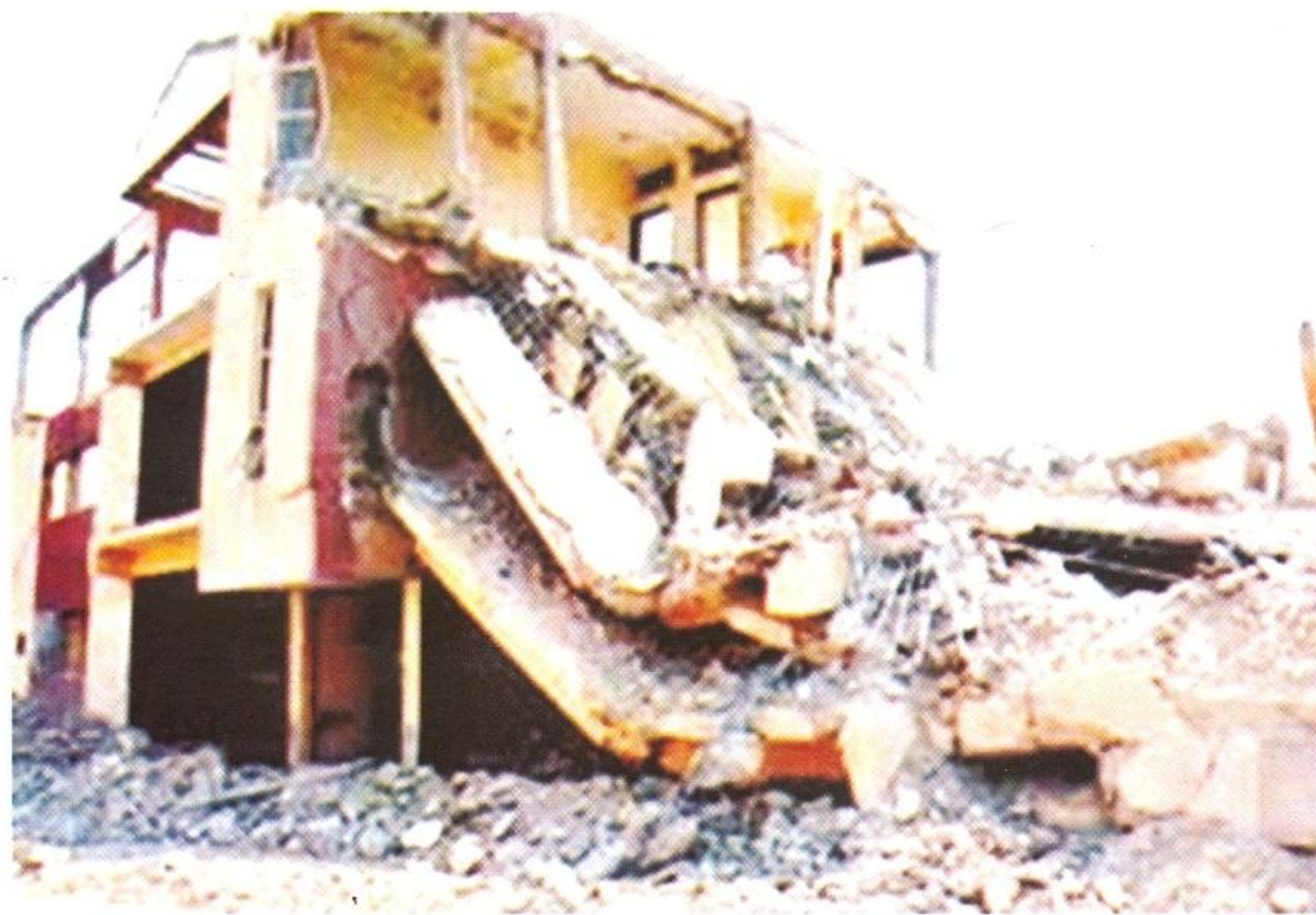
PLATE 6: COLLAPSE OF A TWO STOREY BUILDING OWNED BY NIGERIAN NAVY IN GWARIMPA, ABUJA
