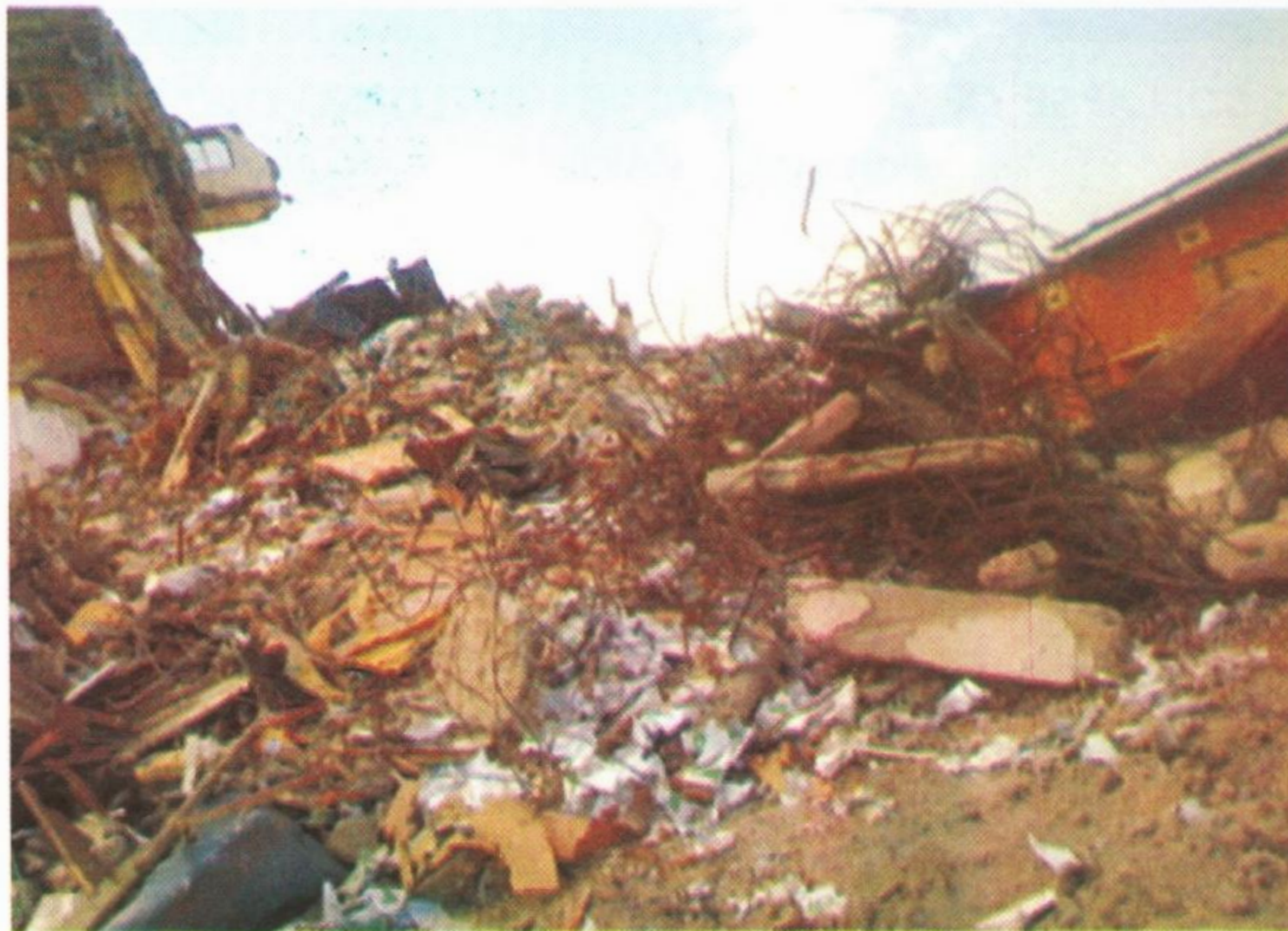
PLATE 5: COLLAPSE OF 6- STOREY BUILDING IN 11 ADERIBIGBE STREET, MARYLAND, LAGOS
