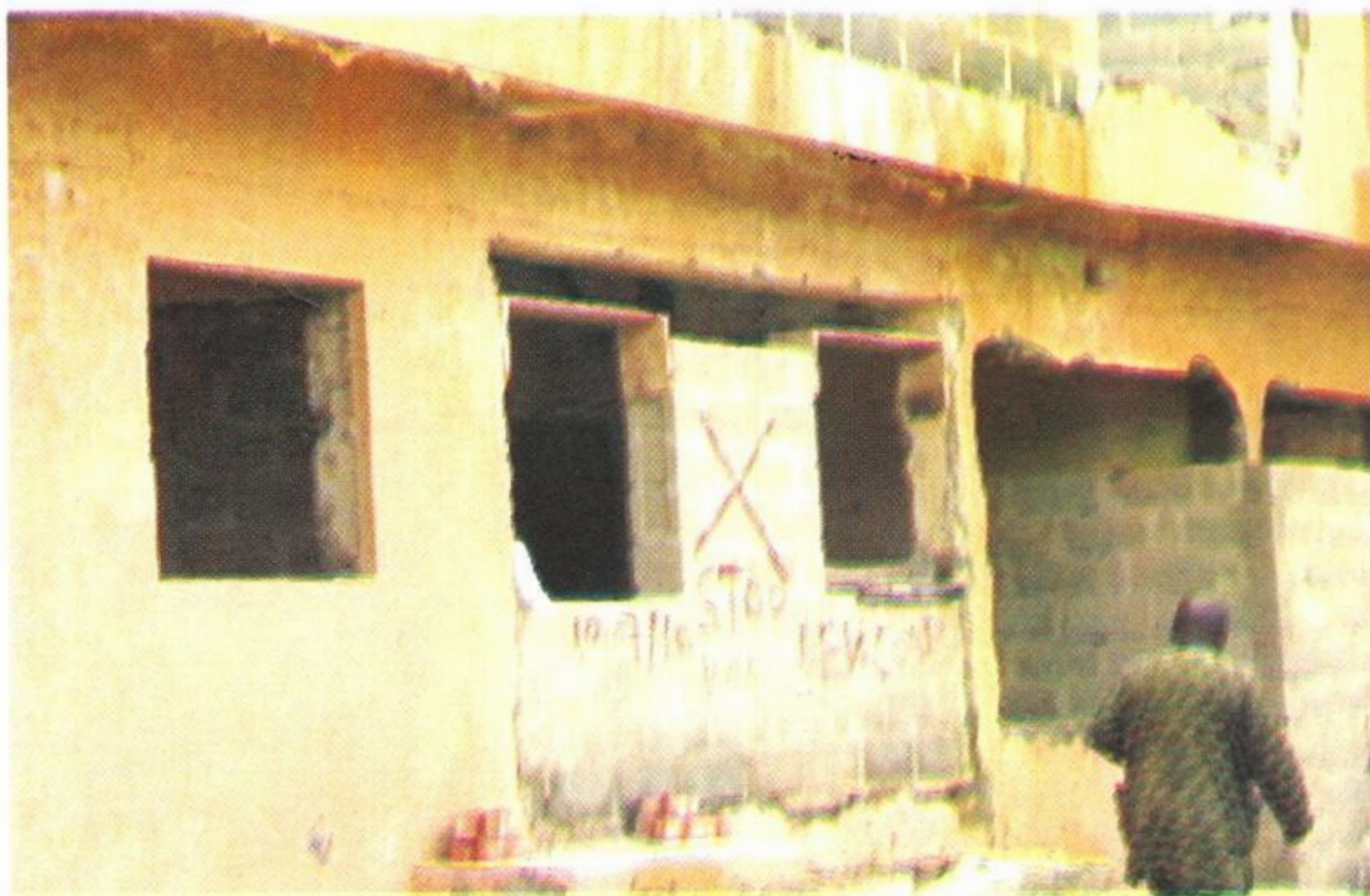
PLATE 11: DEVELOPER INCREASING THE HEIGHT OF BUILDING WITHOUT RECOURSE TO THE AUTHORITY
